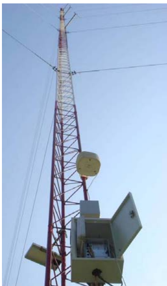
Figure 3. View of 45 m lattice met tower showing data logger and instruments.
